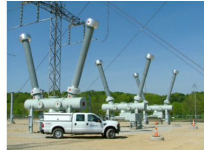
Don Marquis Substation, 800-kV Circuit Breaker's Photo: US DOE
